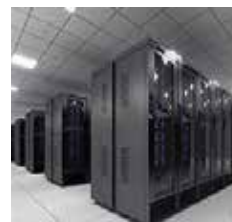
Telecom/IT and Data Centres
